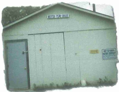
Mester Pump House
